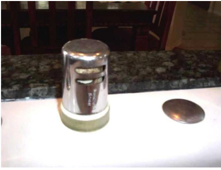
Figure 1. Dishwasher air gap at kitchen sink.
