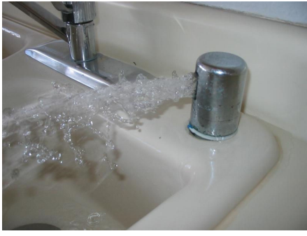
Figure 2. Dishwasher draining improperly through air gap.
